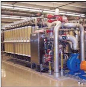
Ultrafiltration Stage on Train #2
