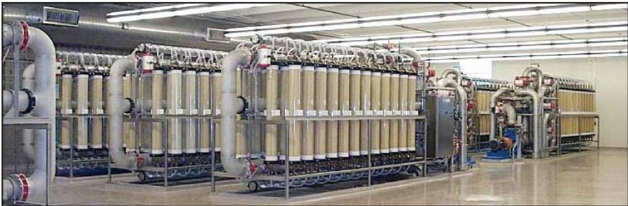
View of Five Ultrafiltration Stages, Train #2
